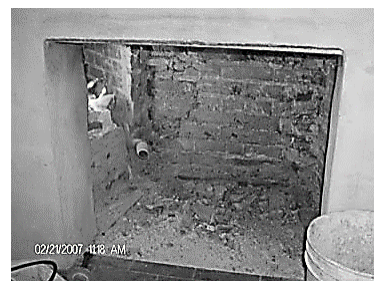
Badly Deteriorated Firebox
