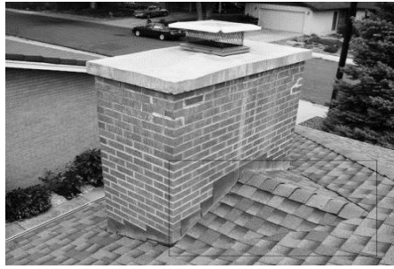
Clay Liner Cover
